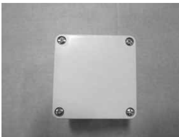
SRV2326-304 Junction Box Assembly
